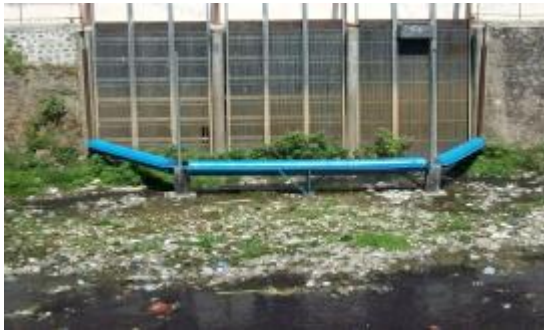
Gambar 28. Trash Rack Manual
